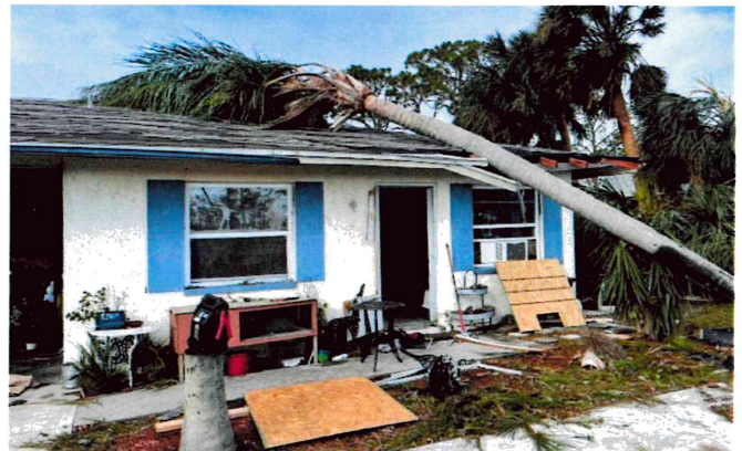
Cheyenne Prevatt's home was damaged by Hurricane Ian and by a fallen palm tree, making it uninhabitable, in Englewood, FL
